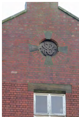
Fig.243 Inappropriate cement pointing
