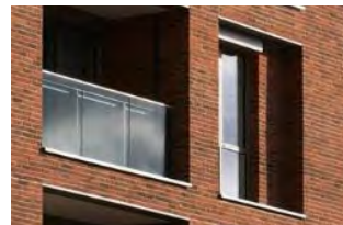
Glass balustrade in the same plane as windows ✓
