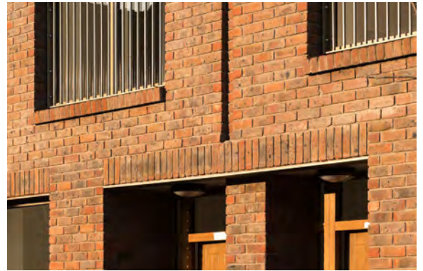
Example of cill and head details, and brick recesses used to articulate brick facades
