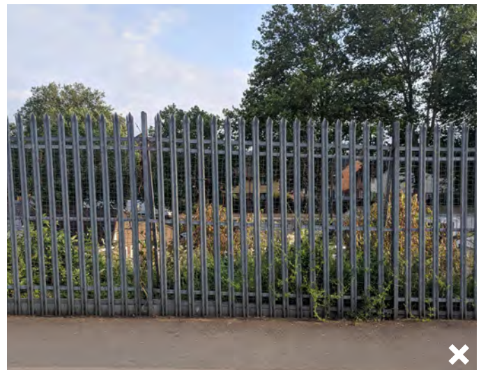
Fig.382 Palisade fencing is un acceptable. Raw steel/metal finishes are not appropriate
